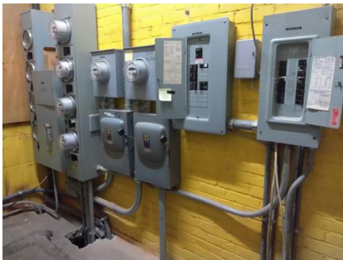
FIGURE 16: ELECTRIC SERVICE AND PANELS - REQUIRE RELOCATION AND UPGRADES
