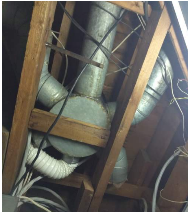
FIGURE 18: BATHROOM EXHAUST DUCTS AT UNDERSIDE OF ROOF JOISTS.
