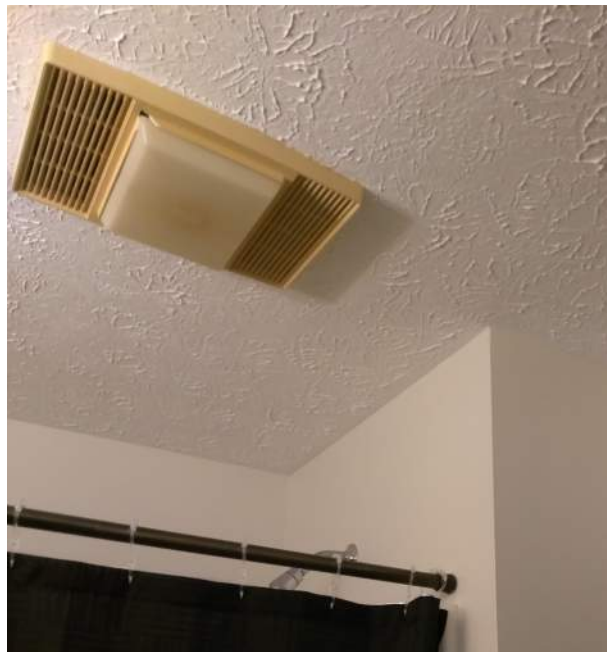
FIGURE 11: BATHROOM EXHAUST FAN WITH LIGHT NEEDS REPLACEMENT, TYPICAL
