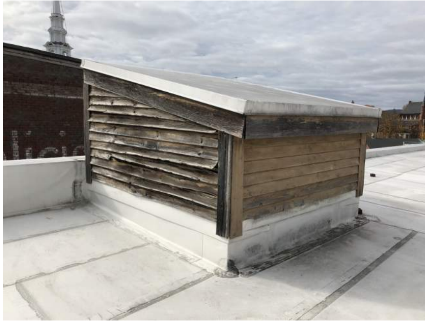
FIGURE 17: ELEVATOR PENTHOUSE NEEDS TO BE REBUILT AND INSULATED.
