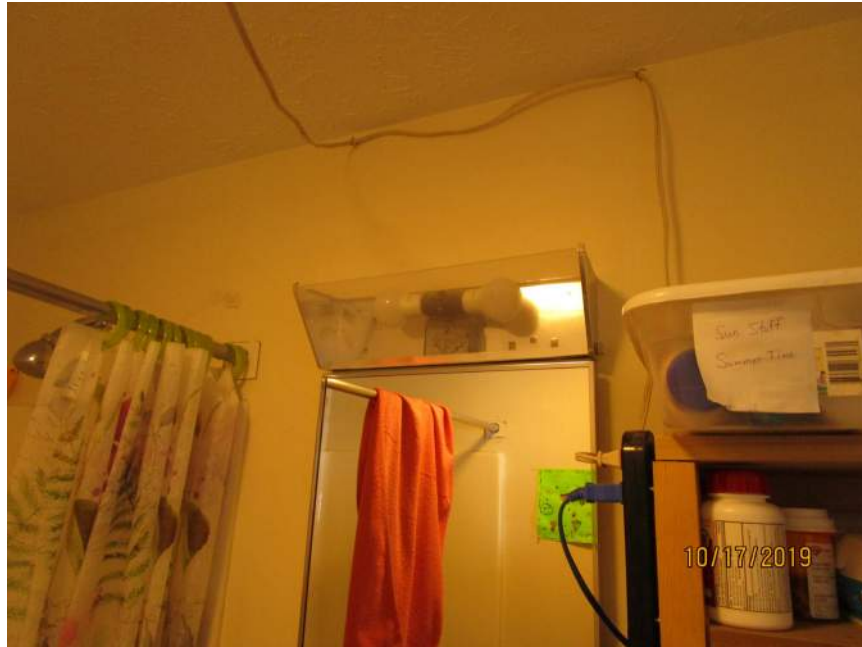
FIGURE 10: BATHROOM VANITY FIXTURE NEEDS REPLACEMENT, TYPICAL
