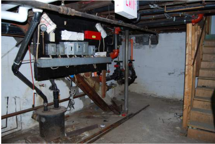
FIGURE 14: ELECTRIC FEEDER PANELS IN BASEMENT NEED REPLACEMENT
