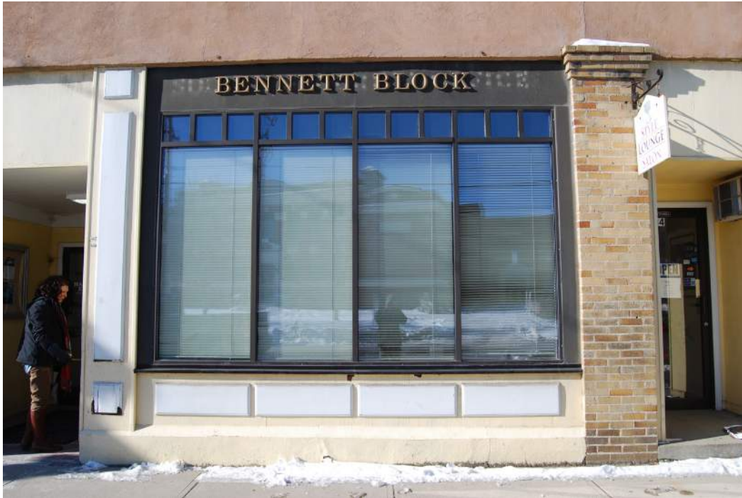
FIGURE 5: STOREFRONT - NEEDS REPLACEMENT AND REPAIRS TO WOOD TRIM
