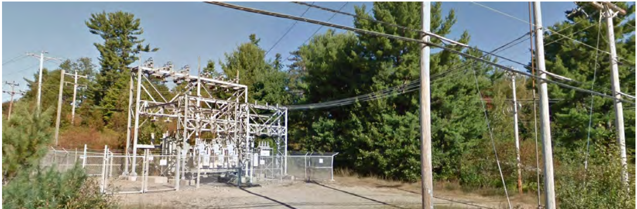
64 Figure 2: Loudon Non-Bulk Station, Loudon NH
