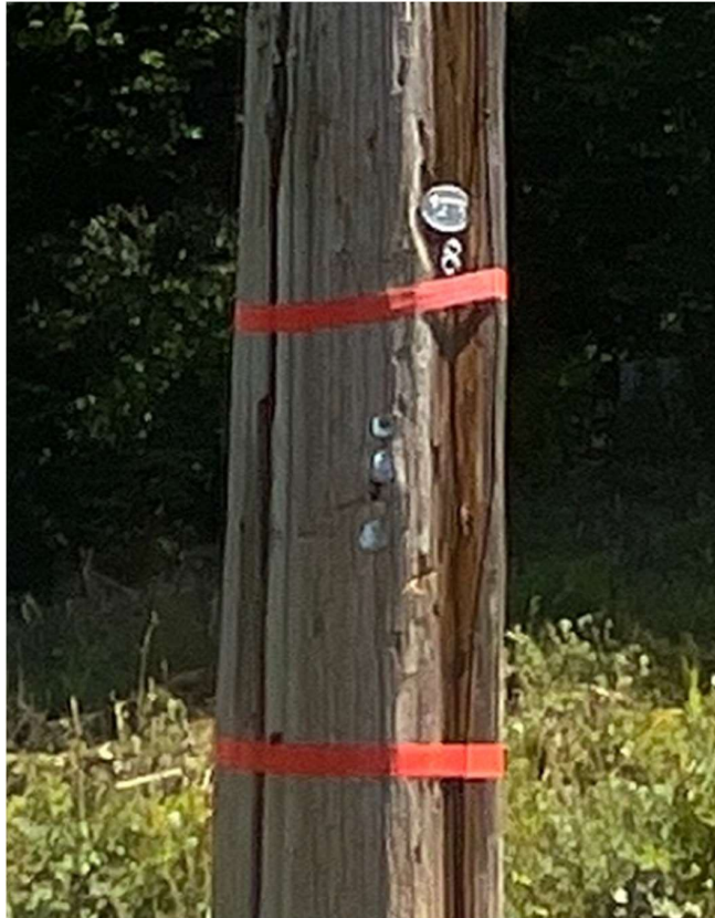
Structure 8 – Severe Structure Splitting
