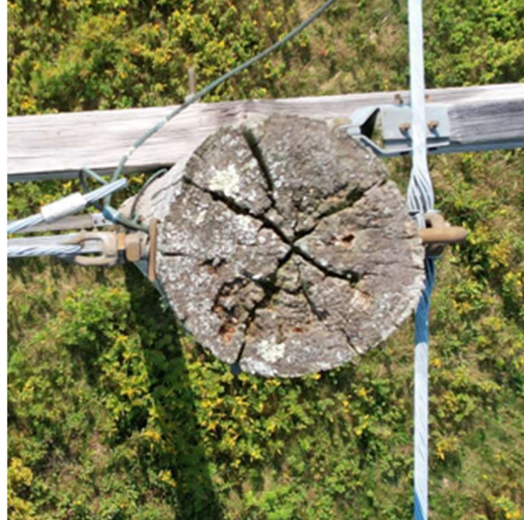
Structure 356 – Split Pole Top
