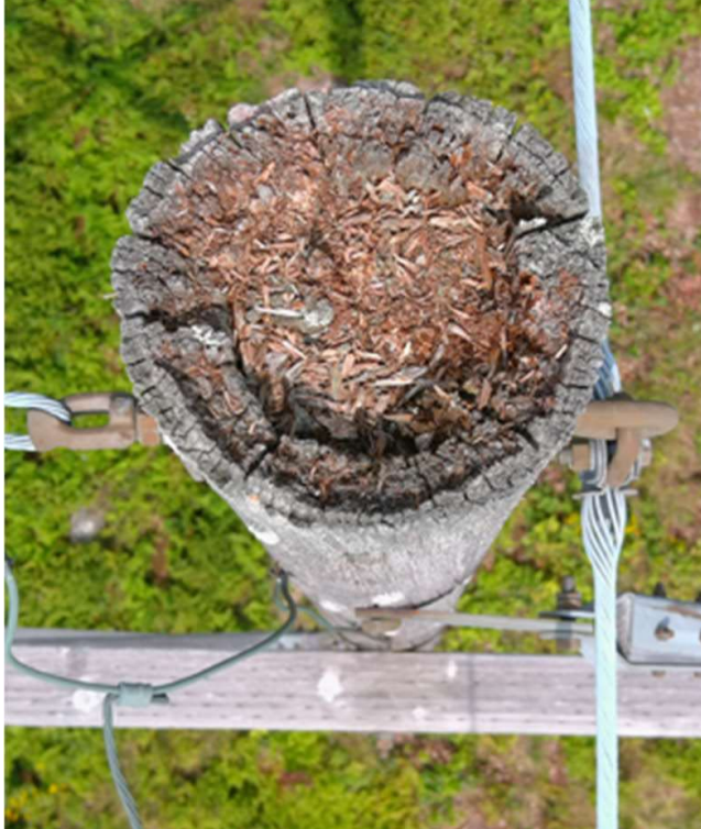
Structure 212 – Pole Top Rot & Rusted Hardware
