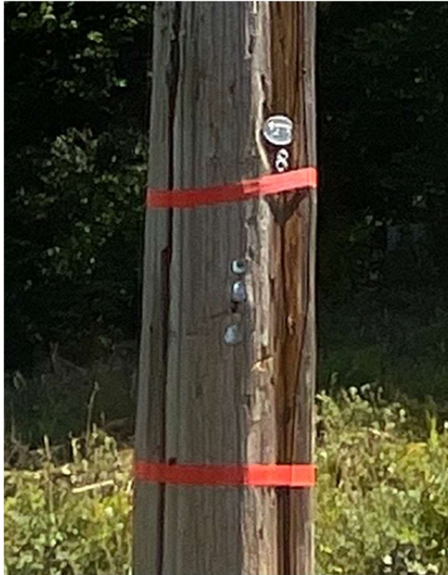
Structure 8 – Severe Structure Splitting
