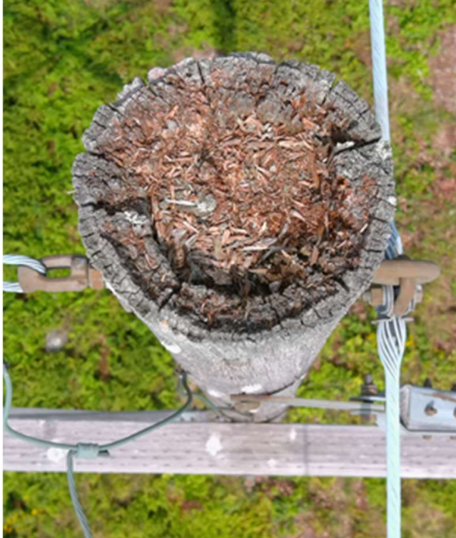
Structure 212 – Pole Top Rot & Rusted Hardware
