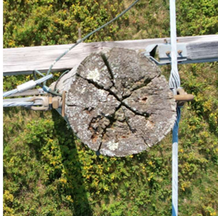
Structure 356 – Split Pole Top
