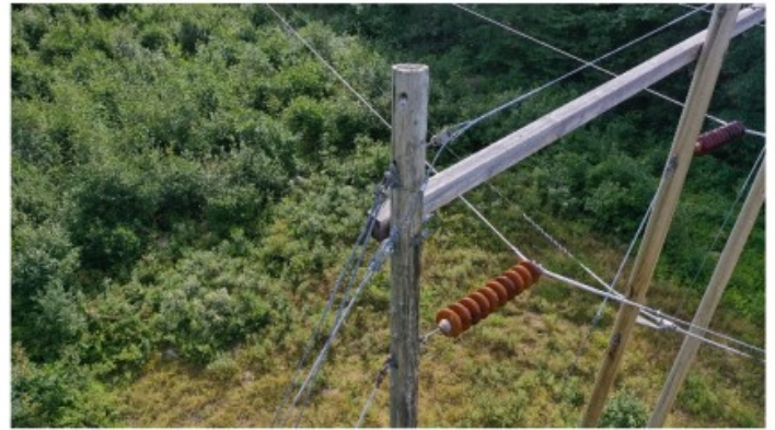
Pole Split – Structure #95
