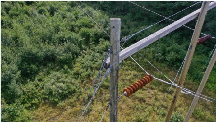
Pole Split and Woodpecker Damage – Structure #205
