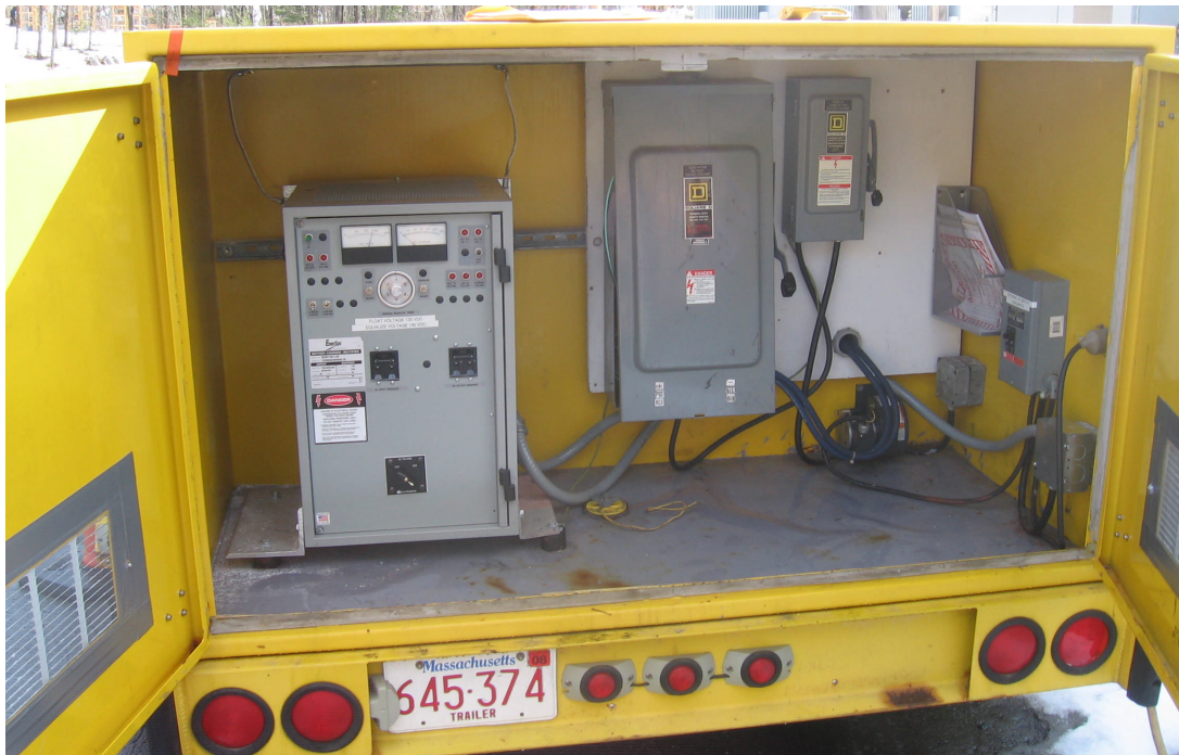
Figure 1 - Typical Battery Trailer Arrangement in Connection Cabinet
