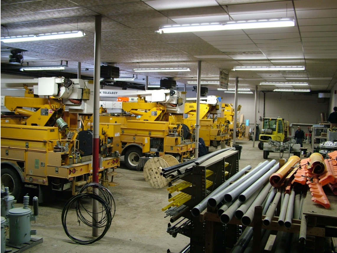
Figure 1b: Portsmouth AWC Garage Lighting (After EE Upgrade)
