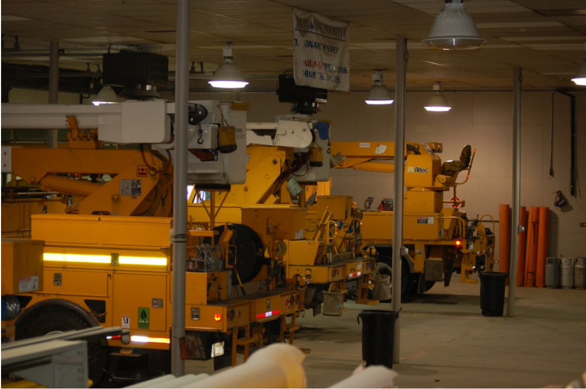
Figure 1a: Portsmouth AWC Garage Lighting (Before)
