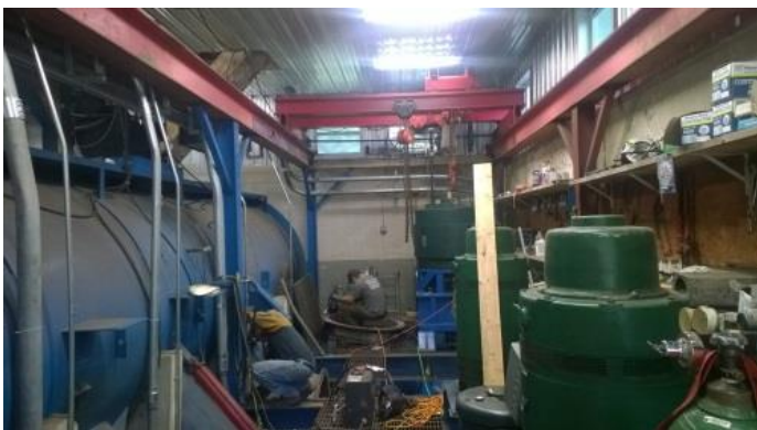
Steels Pond Hydro
