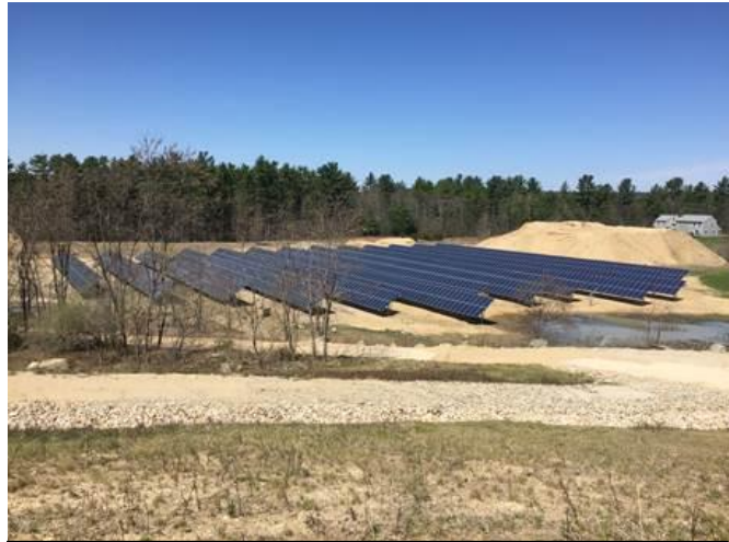
Durham Solar Project
